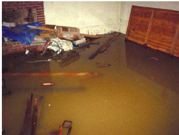
Photo 8. Excess moisture during construction can leave mold growth.
