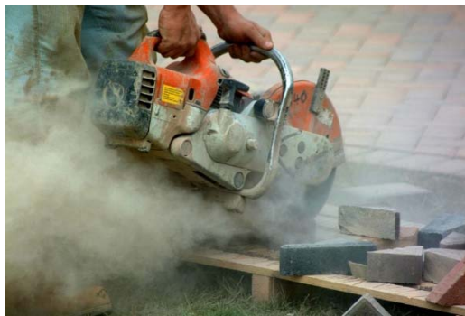
Photo 5. Construction tasks with the heaviest emissions may need to be restricted to after-hours.
