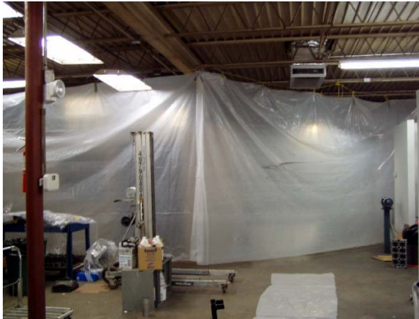
Photo 4. Dust curtains may be insufficient to prevent contaminant migration.
