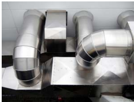
Photo 7. Air supply and return systems work areas should be sealed off from occupied space.
