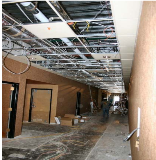
Photo 2. Pathways from work areas include openings, penetrations, air intakes and foot tracking
